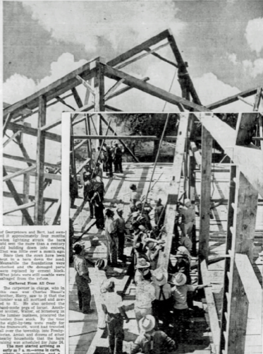
ALL-OUT JOB was getting the putties to the floor at last week's barn raising down at Green Tree. Most step was getting it up into the rapidly developing structure. With plenty of team work and chomped grass, stanchions (guiding poles), and ropes, the putties which helped form the frame of the barn were eventually nailed into place. By noon the completed barn's skeleton was outlined against the sky.
