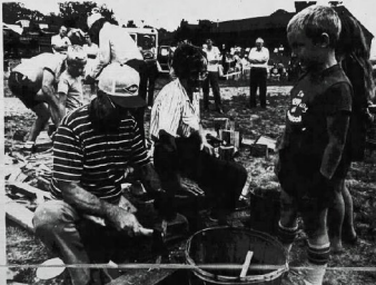
Eugene Schertz of Metamora (left, with hatchet) carved wooden pegs while his wife Optra (second from left), his grandmother Anne Schertz of Metamora (partially obscured) and Jed Wullmar of Goshon, Indiana (right) look on. The pegs were used to hold the barn beams together, just as the barn was constructed originally 124 years ago.
