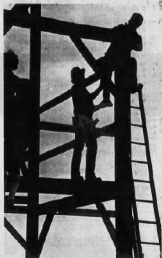
Volunteer laborers from all over Central Illinois, and a few from out of state, helped assemble the barn. Pictured are two workers fitting together beams at the corner.
